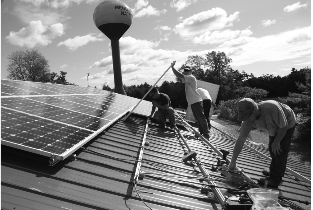
A work crew installs solar panels on a building at the College of Menominee Nation's (CMN's) Keshena campus to support applied research by CMN faculty, engineering students, and others engaged in the College's Solar Energy Research Institute. (Photo credit: CMN by DKakkak)
