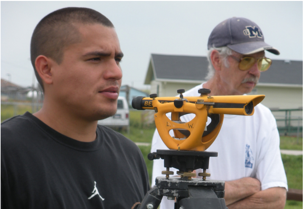
Willis Zephier, Oglala Lakota College PEEC student; and South Dakota School of Mines & Technology faculty member, Dan Dolan, surveying the building site for a sustainable greenhouse on the Pine Ridge Reservation in South Dakota. (Photo credit, J.F. Sawyer)
