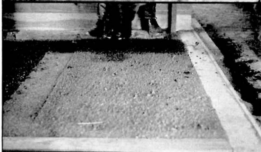
Fig. 12. Sprinkling the cut-back asphalt oil onto the loose soil mixture from an old can with perforated bottom. The worker must stand on a plank in doing this.
