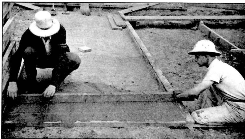
FIG. 8. STRIKING-OFF THE LOOSE SOIL-CEMENT MIXTURE BEFORE RAMMING IT FOR THE TOP COURSE.
