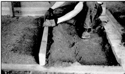
Fig. 11. Striking off the loose soil mixture for the top course with straight-edge, ready for the oil.
