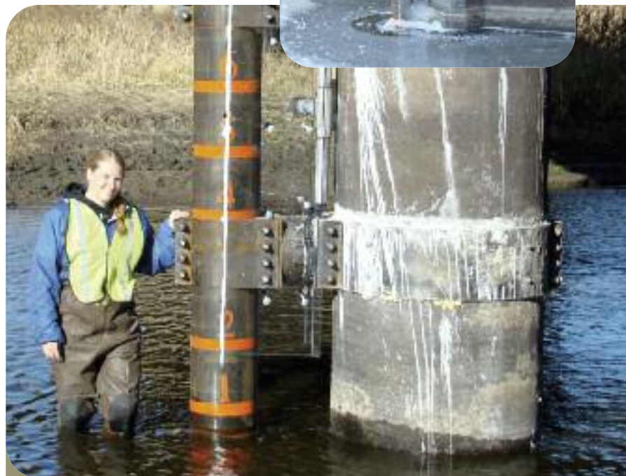
Top: Ice hugs a bridge pier and an attached measuring device in the James River east of Huron. The device is used in a project to calculate ice load.
