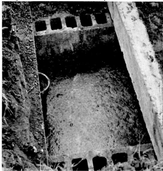
Fig. 4. Block tank in use for four years
