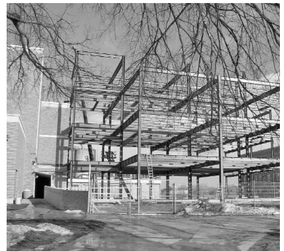
In March the steel skeleton suggested just how large the building is going to be.
