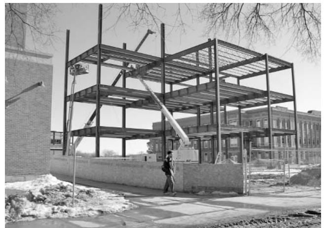
In February lots of steel beams could be seen above the foundation.
