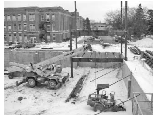
After much underground preparation and pouring of concrete for the foundation, January saw work begin above ground.
