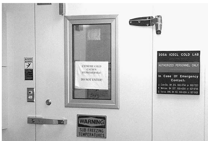
Exterior of the twenty-by-ten foot walk-in freezer in the ice core and environmental chemistry lab (ICECL).
