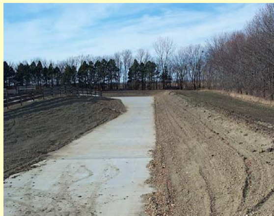
Constructed first phase of an Animal Waste Management System designed by USDA/NRCS
