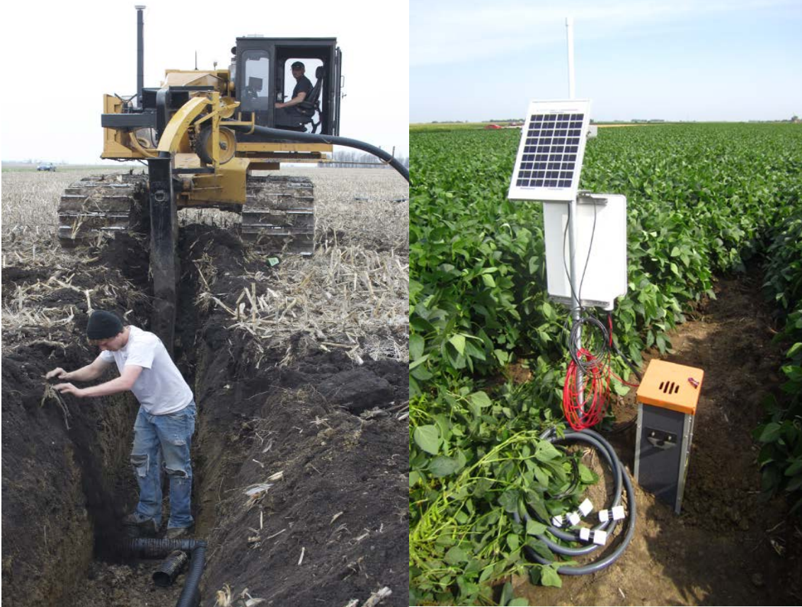
Photos of drainage installation and plot control structure and monitoring instrumentation.
