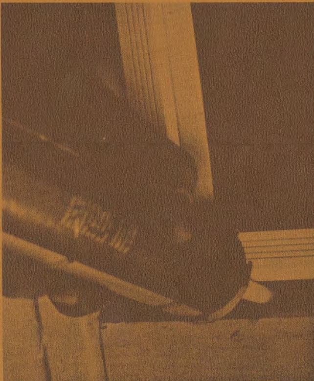
When caulking with a gun, hold the gun at a 45° angle and slant it in the direction of movement.
