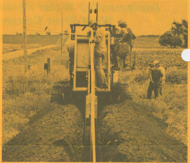
Construction of a rural domestic water supply through a community water system project in Lincoln County.
