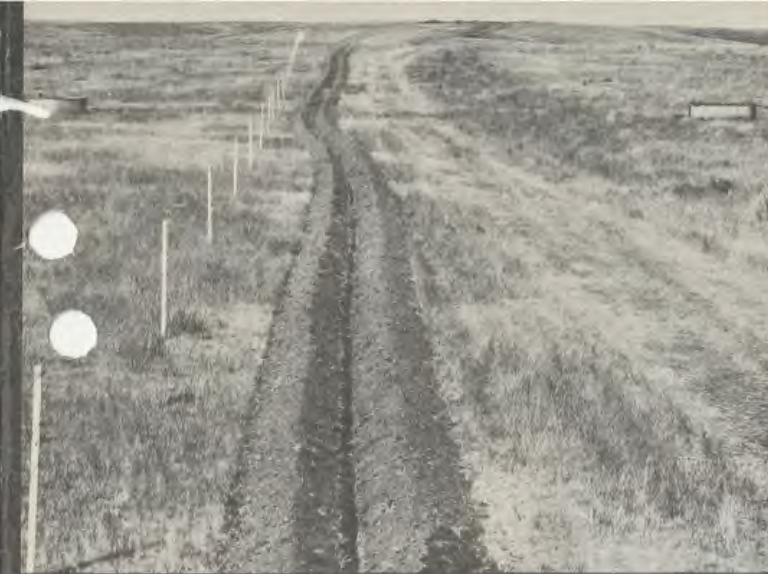
Practices include pipelines which may distribute water to several pastures, thus reducing water cost per acre.
