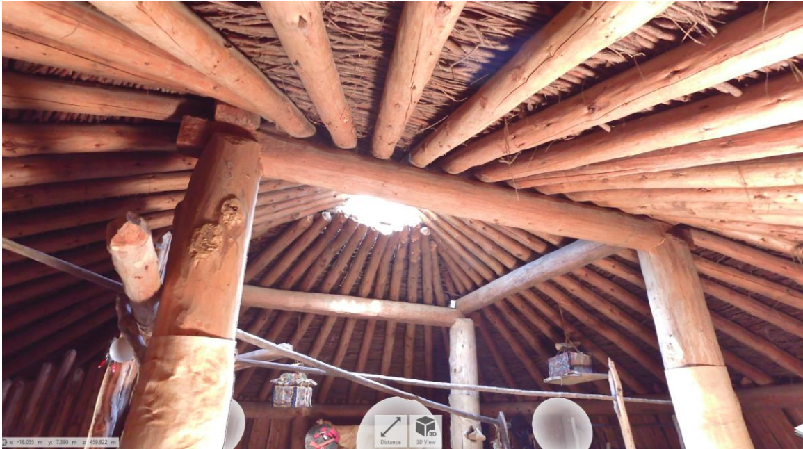
Figure C-3. Final rendering obtained from Autodesk Recap 360, showing detail of roof beams of the reproduction earth lodge at Knife River Villages National Historic Site. This reproduction earth lodge was built based on Wilson's (1934) plans sketched by his associates.
