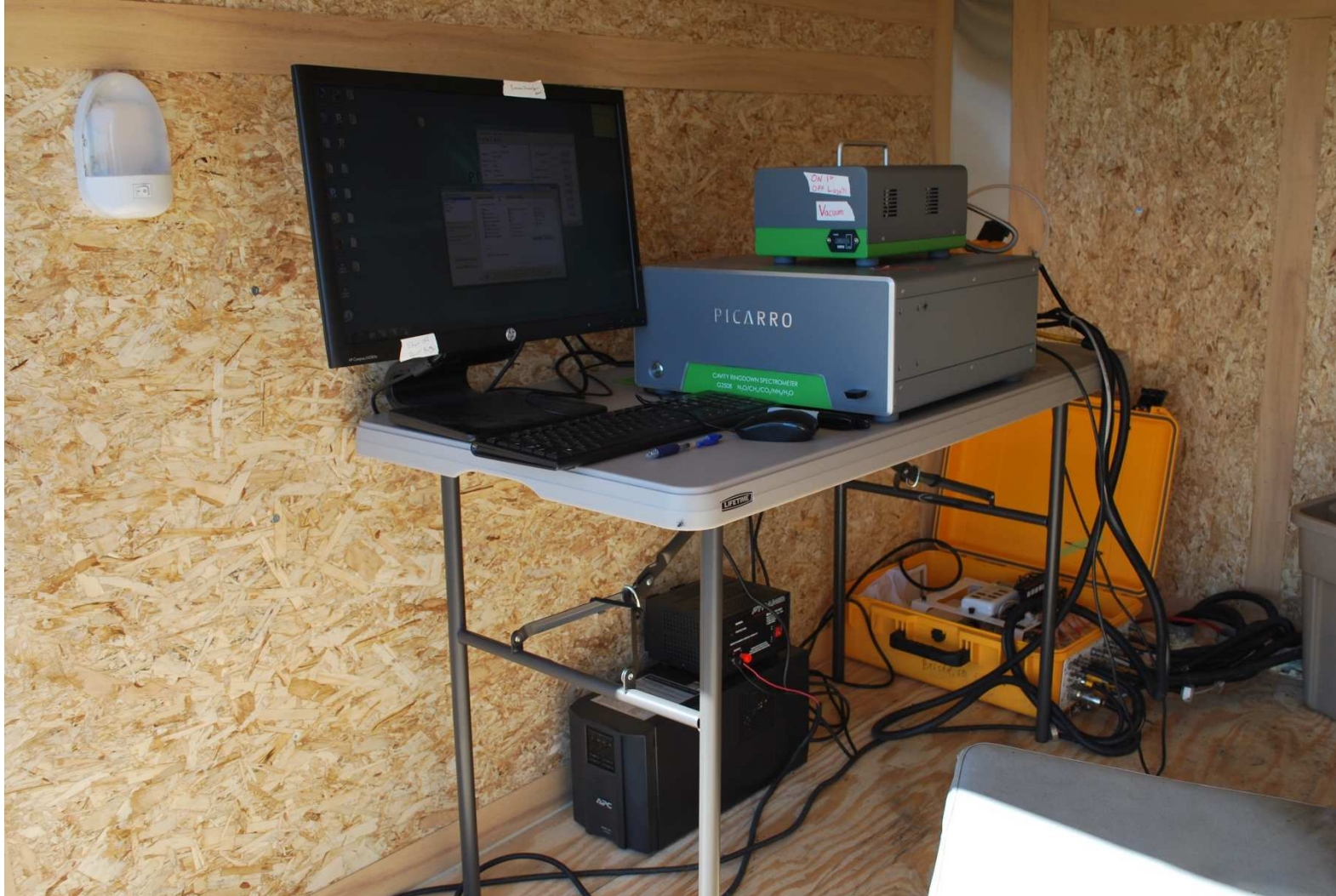
Supplemental Picture 4: This picture shows the inside of the weatherproof trailer. The LI-COR LI-8150 multiplexer is located in the lower right side, the Picarro Cavity Ringdown Spectrometer is located center, and a backup battery and surge protector are located underneath the table.
