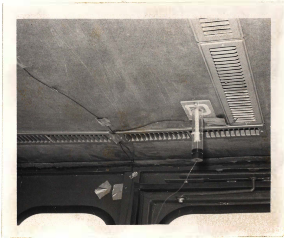
Figure 3. Louvered Air Distribution System
